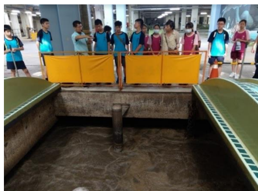
A study visit to the Dihua Sewage Treatment Plant
